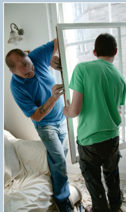
Repairing the sash cords of a timber sash and case window. Most components of a traditional window can be repaired without the waste of replacing the whole unit.
