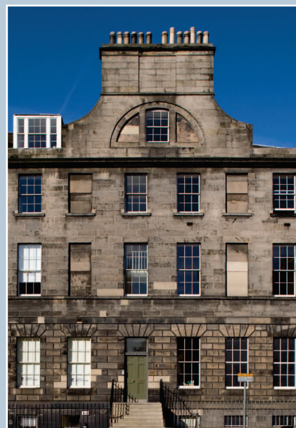
South Charlotte Street, Edinburgh. The blind openings are detailed with sills and a 'meeting rail' to maintain the symmetry of the architectural elevation. The chimney flues pass behind the blind windows. © N. Haynes.
