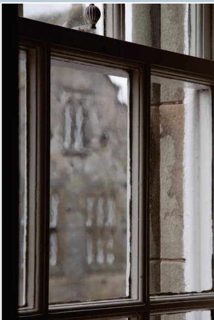
Detail of a timber sash and case window of circa 1890 showing the profile of the astragals, the irregularities of the glass, and a decorative sash fastener. © N. Haynes.
