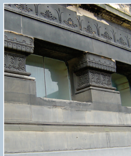
St Vincent Street Church by Alexander 'Greek' Thomson, St Vincent Street, Glasgow. Thomson's Graeco-Egyptian designs emphasised the solid monumentality of the masonry against the void of the window openings. He used large sheets of plate glass and minimal frames to achieve this effect. © S. Dibdin.
