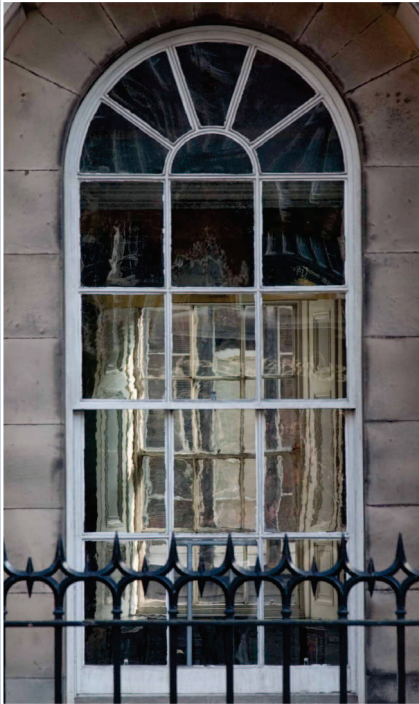
Signet Library, Parliament Square, Edinburgh, circa 1810. A round-headed cylinder glass sash and case window with slim 'astragals', or glazing bars. Irregularities in the glass provide the variety and individuality of the reflective pattern. © N. Haynes.
