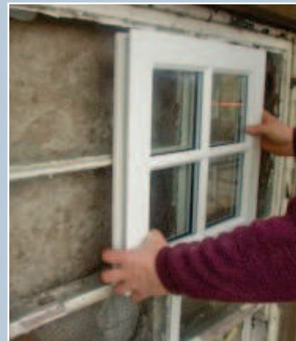
Details of proposed replacement windows should be checked against the originals where possible. In this case the astragal profiles of the sample replacement window are too thick and flat, and would not be an appropriate match for this situation.
